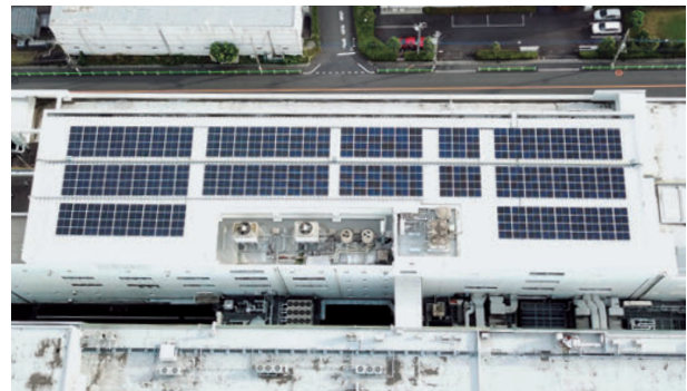
Solar system on roof of Building 3 at the head office
